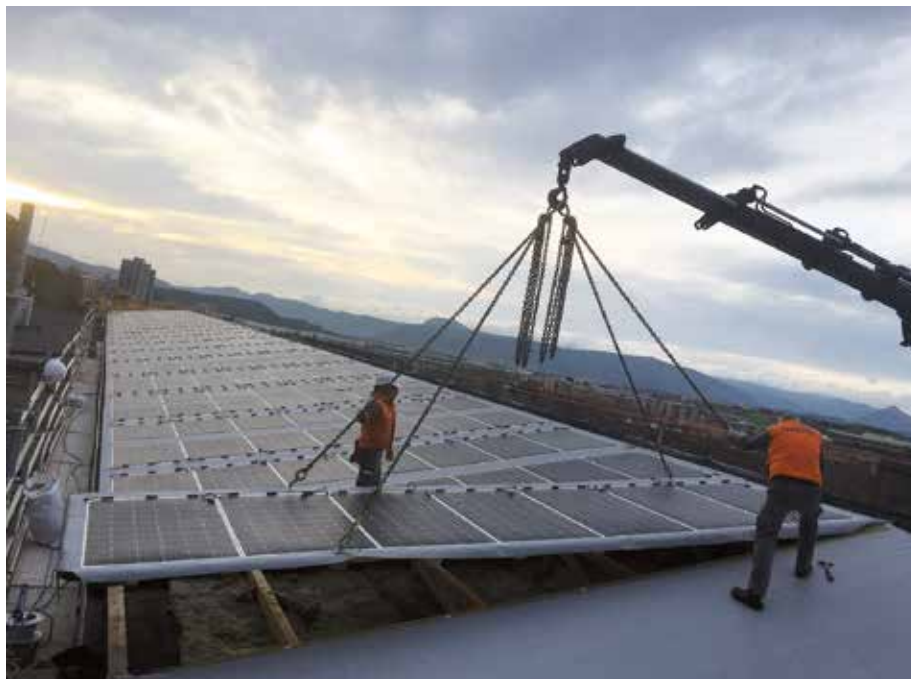
Figure 1: Installation of a prototype Plug&Play solar roof on the Municipal Police building in Pamplona (Spain). The panels will provide energy for self-consumption and are connected to recycled batteries for energy storage
